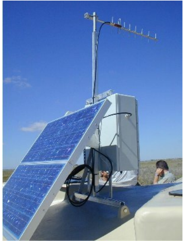
Fig. 5. A detail of a tank top positioned in the field.
